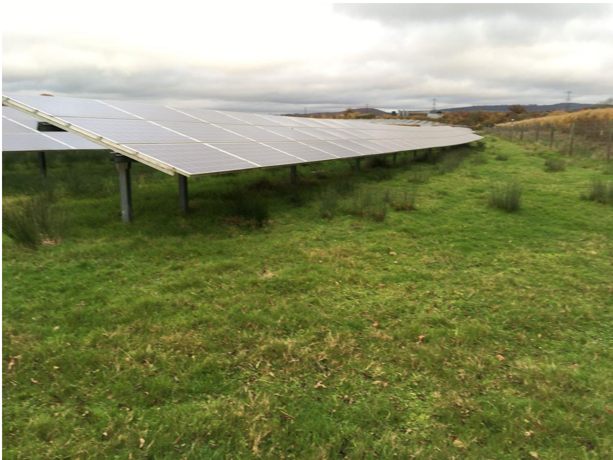
Figure 6-1 Drainage of solar panels onto grass
